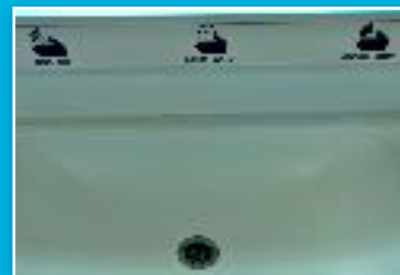
Toilet basins with their own touch taps for water, soap and blow dry
